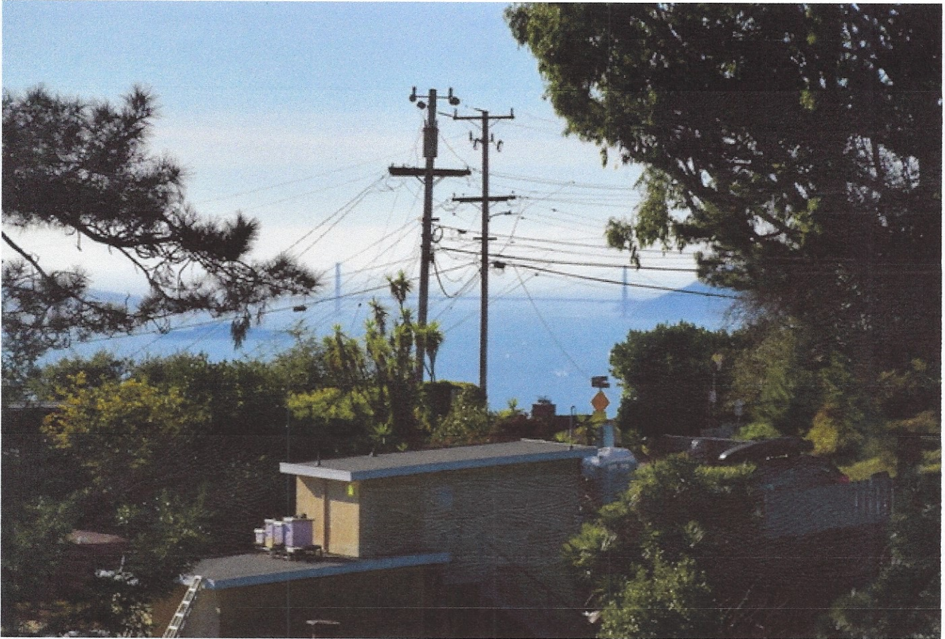
Utility Poles in UUD48, Berkeley CA January 2020
